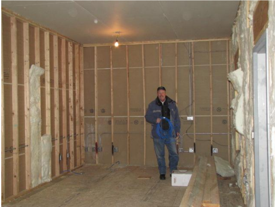
Wiring in the computer room...
